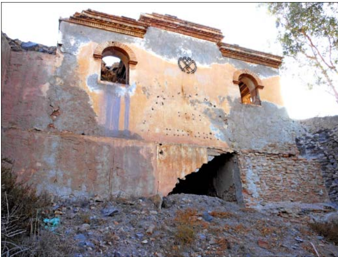
All that remains of the beautiful building that housed Pozo Encarnación.
