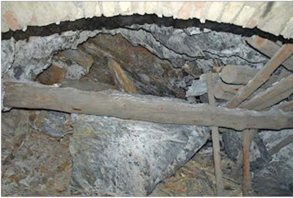
A collapse within the tunnel. Photos A G Jódar.
