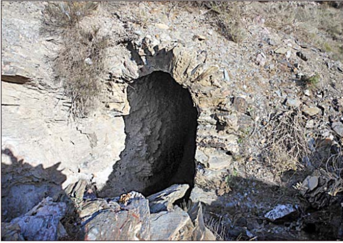
The entrance (above) and exit (right) of the tunnel under Esperanza which channelled the rambla.
